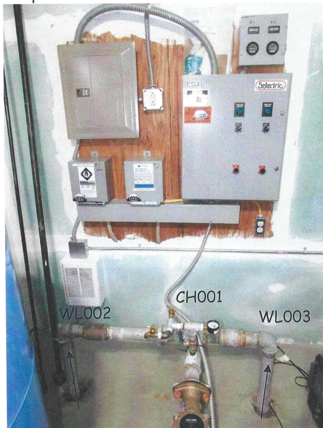
Common Header (CH001) for the wells in the pump house. Well pump control boxes and master controller
