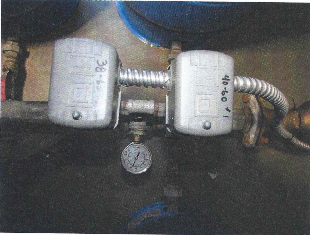
The pressure switches are set to lead/lag pressures of 40 - 60 and 38 - 65 psi.
