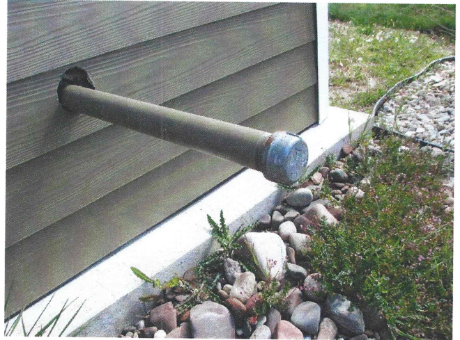
The blow off is capped on the outside of the building.
