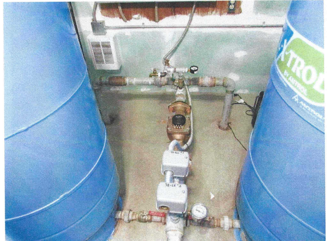
Pressure Control Assembly 1 (PC001) - two pressure switches and 8 Well-X-trol captive air tanks.
