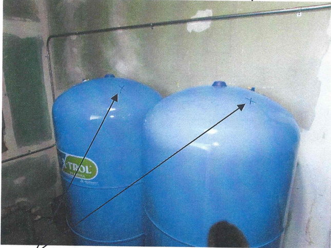
Note the "x" on these tanks showing that they're believed to be waterlogged. They were in the process of being replaced.
